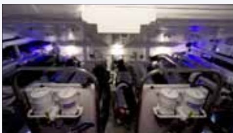
With a camera connected, you can monitor the engine room or get better stern visibility for increased safety.
